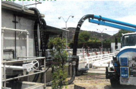
EPCE has extensive experience with the City of Stanton performing pipe cleaning and CCTV inspection.
